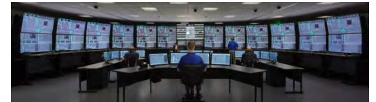
NuScale Control Room Simulator
